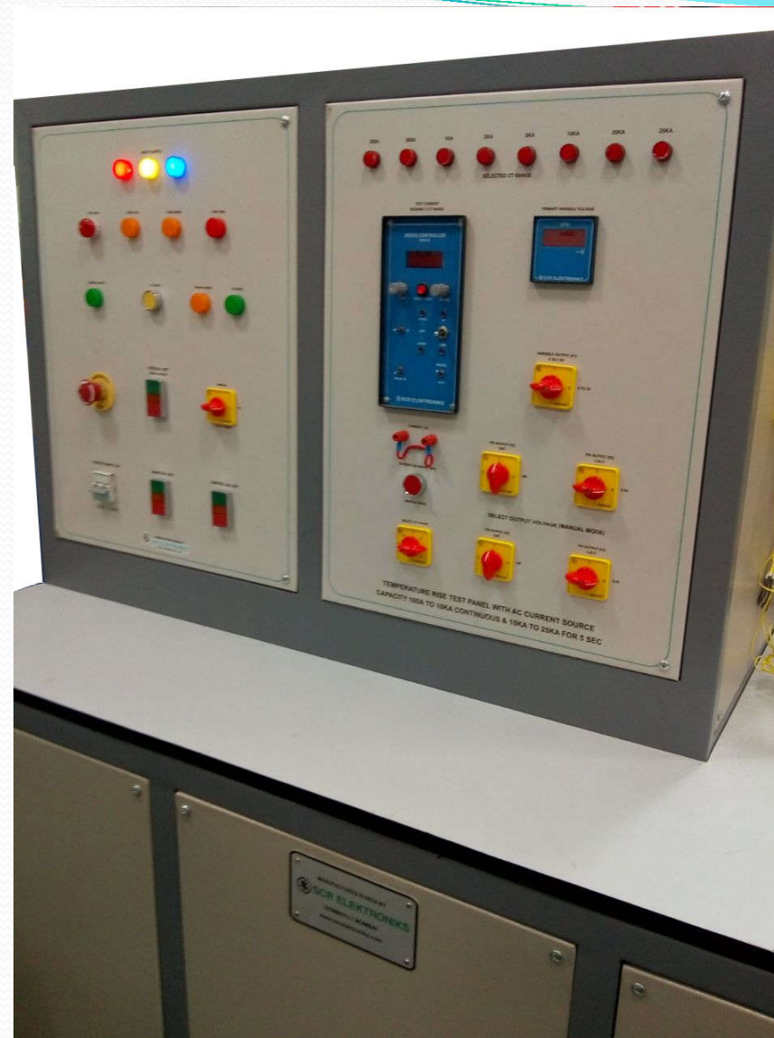
Temperature Rise Test Panel 25kA
